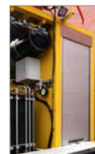
Roller door for hydraulics unit
